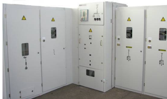
Figure 6. Configuration of Medium Voltage Cells and Corner Connection Due to Limited Space in the Station
